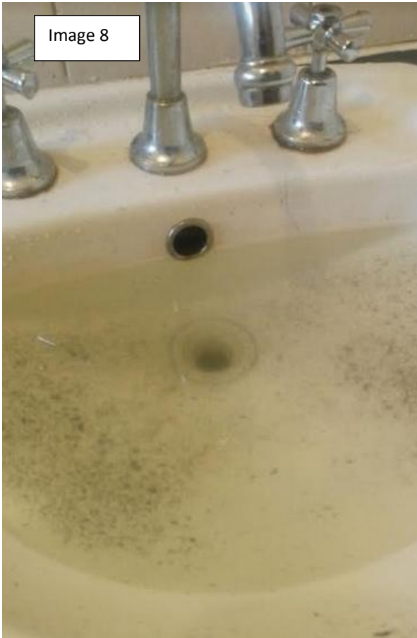
Permanently blocked bathroom basin
