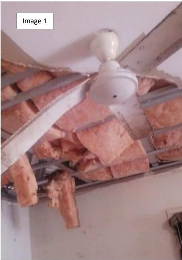
Ceiling fan damaged from ceiling collapse
